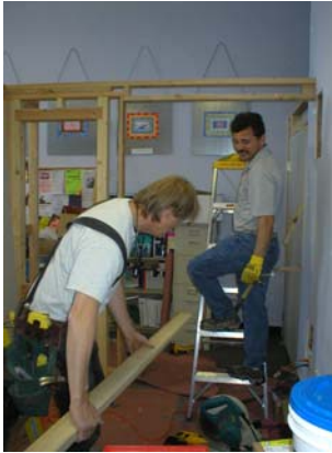
Meet the contractors! Pictured above are lead contractor, Paul Porter (background) and his assistant, Dave Behnken (foreground) of Construction Services, Department of Public Works, County of San Mateo. Not pictured, Val Vaillancourt, electrician.
